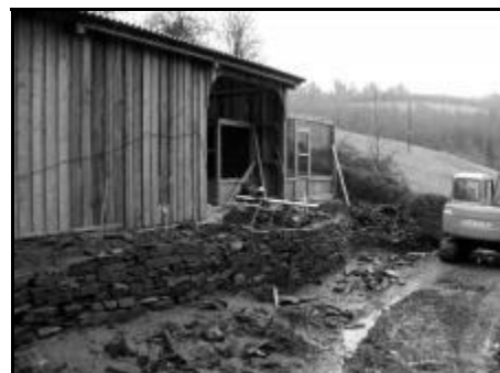
By the 3rd March the wall was well underway and then it rained.... Actually it poured. However we were still on schedule for completion. â
