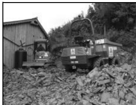
It wasn't long before they hit bedrock and had to bring a rock breaker in. This was really noisy but fortunately didn't go on for too long. â
