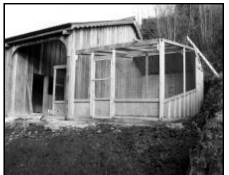
All of the materials had to be carried up the uneven slope. By December the wire
