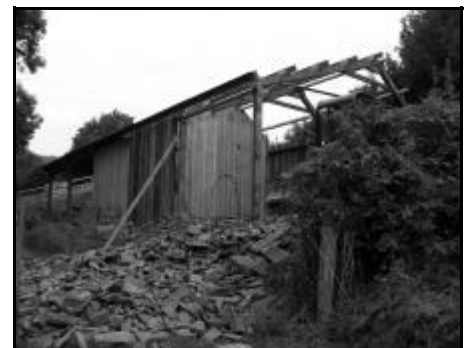
The rock was moved, sorted by staff and volunteers and stored for later use. Once the site was cleared the building went up really fast. æ
