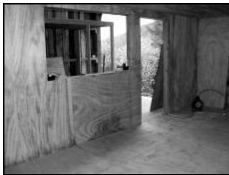
The hospital was a dark ply lined room that needed to become a bright, light and easy to clean space. â
