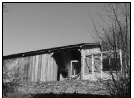
5th March - almost there now just the access path, fence and a few other finishing touches to do before the birds can move in. ç
