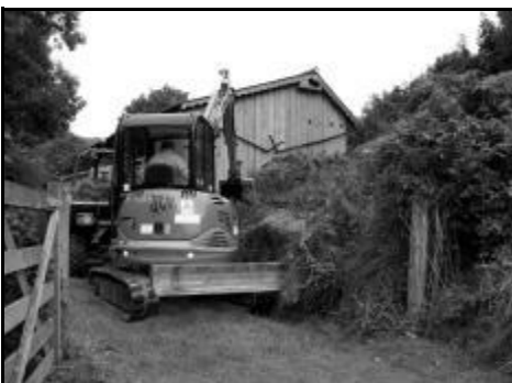
This end of the barn was where the extension would go. Before construction could start the site had to be cleared .
