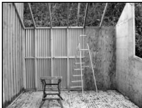
The back was covered with corrugated sheet and then lined with FSC ply. The back was also roofed. â
