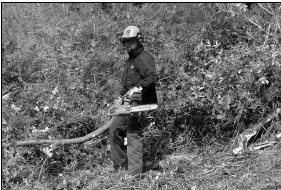
Matt clearing scrub to enable us to build the hedgebank and stone wall
