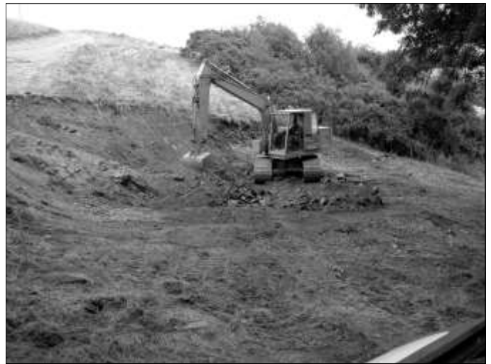
Creating a space for our new barn. We used the soil to create the new hedge bank
