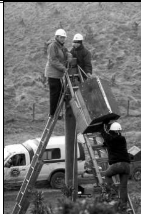
Pole box erection - Conservation workers Mark Green, Sue Searle and Amy Oliver take the strain. Photo: David Ramsden
